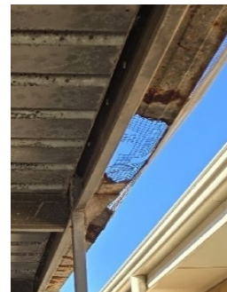
Rusted and damaged gutter.
