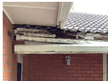
Dislodged and rusted gutter.
